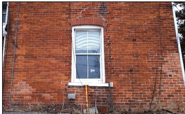
Plate 13: Detail of existing condition of exterior bricks and windows
