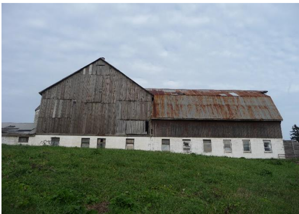
Plate 20: West elevation of the barn complex showing bank barn (left) and gambrel addition (right) (Town of Oakville 2014).
