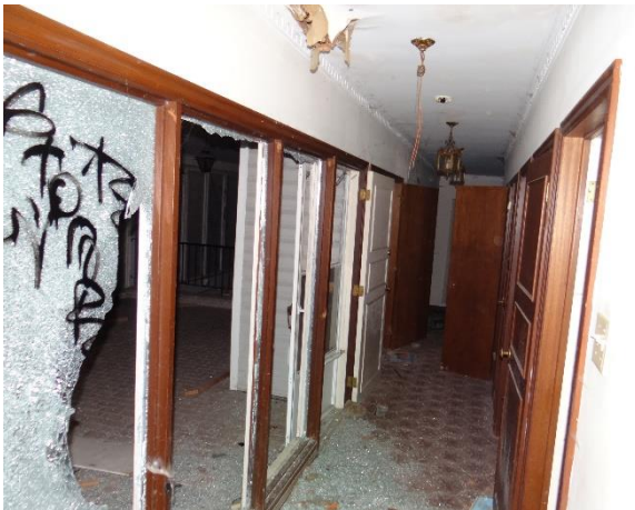
Plate 24: Looking east along hallway, patio door is on the left, bathroom/kitchen doors on the right
