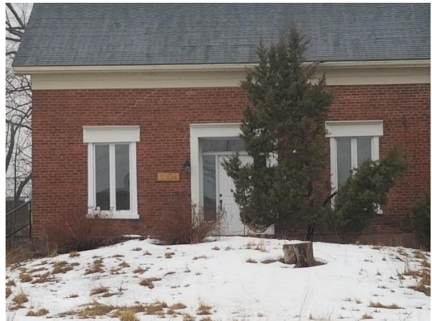
Plate 9: Detail of front elevation, replaced windows, and vinyl fascia under the eaves (March 2020)
