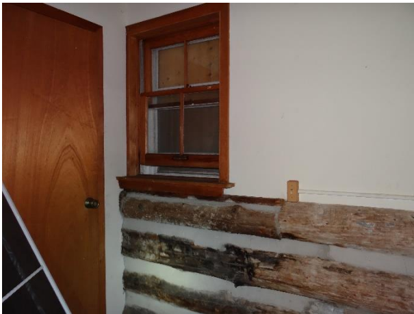
Plate 16: Detail of the logs and window on east wall of the hallway, log house second floor
