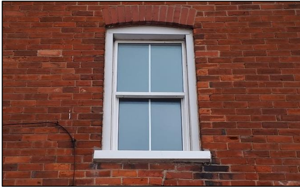
Plate 14: Detail of vinyl window replacement and (likely) vinyl or aluminum capped frame and sill. Brick deterioration is also observable
