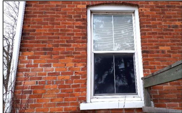
Plate 15: Detail of vinyl window replacement on primary (east) elevation and repointed and spalling brick (left)
